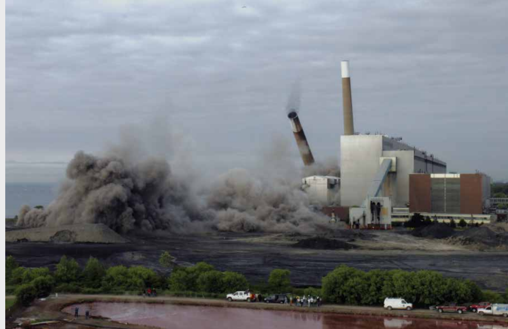
Lakeview Coal Plant demolition, June 12, 2006. PHOTO: LAWRENCE R. NICOLL. COURTESY MISSISSAUGA LIBRARY SYSTEM.
